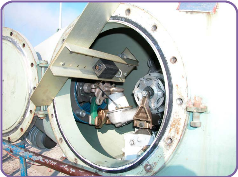
Figure 29. Westinghouse SFA Transducer Installation
