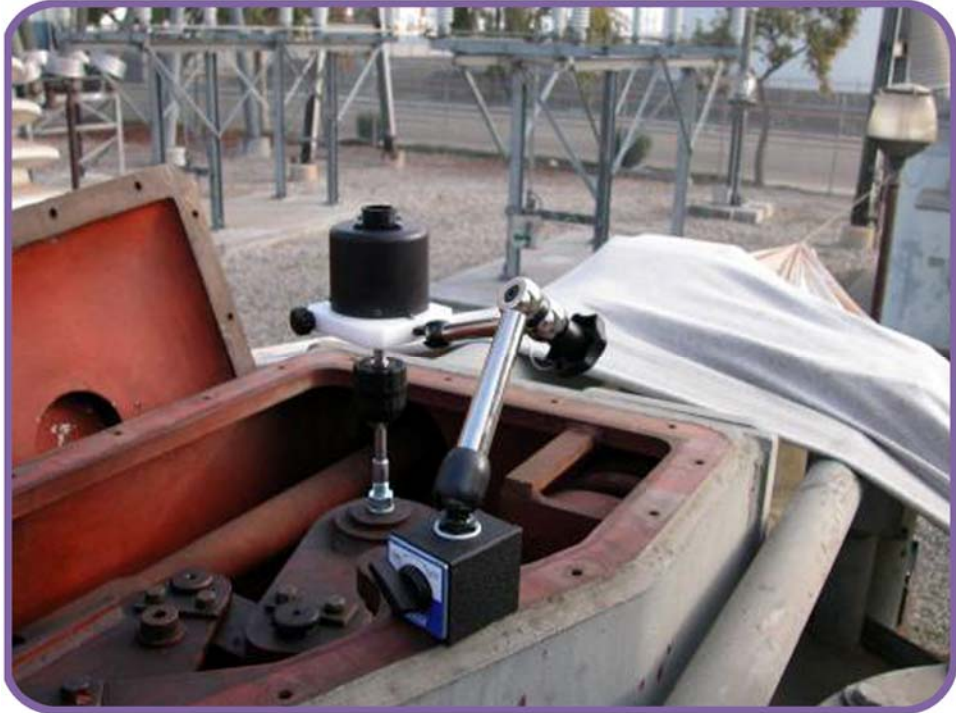
Figure 32. Rotary Transducer on Federal Pacific Breaker
