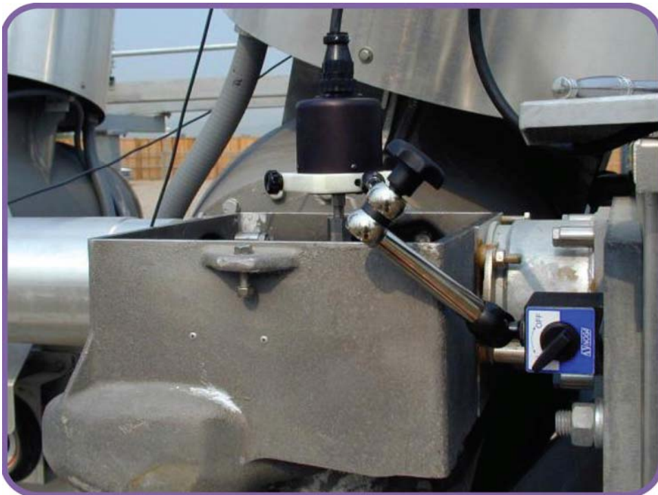
Figure 27. Rotary Transducer on Alstom HE 1014 Circuit Breaker
