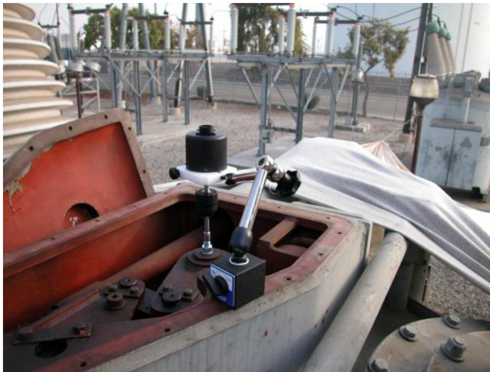
Rotary Transducer on Federal Pacific Circuit Breaker
