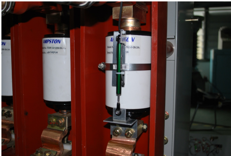
Resistor Transducer on Vacuum Circuit Breaker
