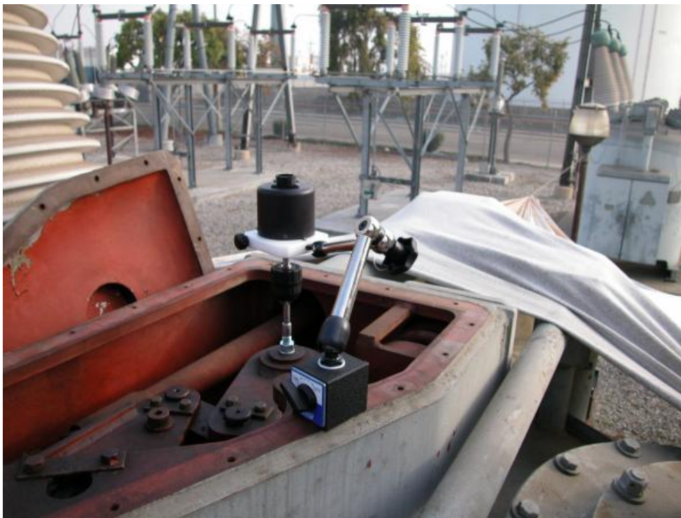
Rotary Transducer on Federal Pacific Circuit Breaker
