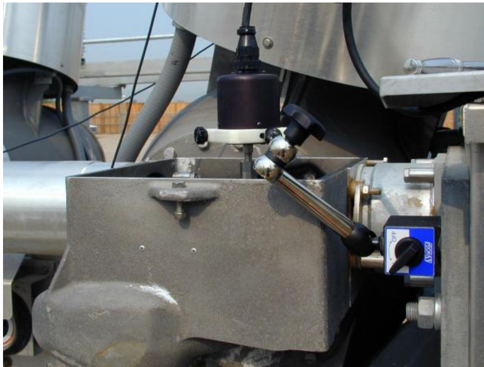
Rotary Transducer on Alstom HE 1014 Circuit Breaker
